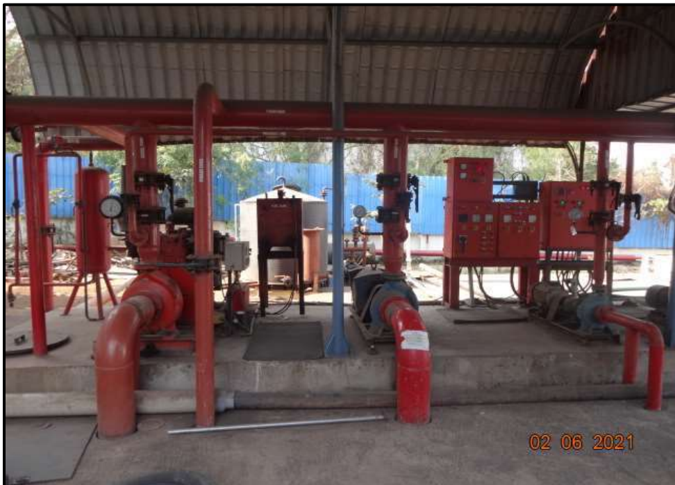
Fire hydrant tank & pumps
