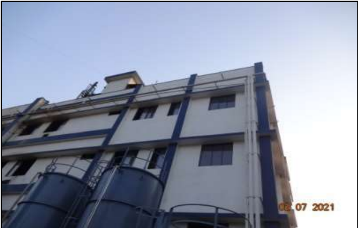
Rain water harvesting pipeline from Terrace
