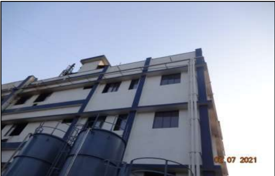
Rain water harvesting pipeline from Terrace
