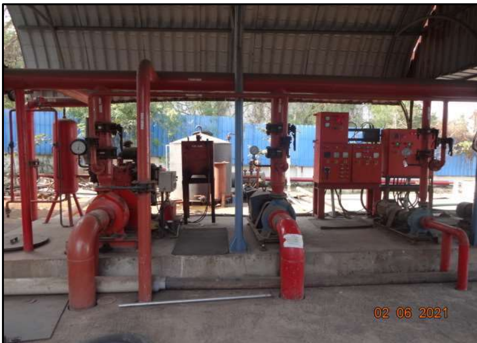
Fire hydrant tank & pumps
