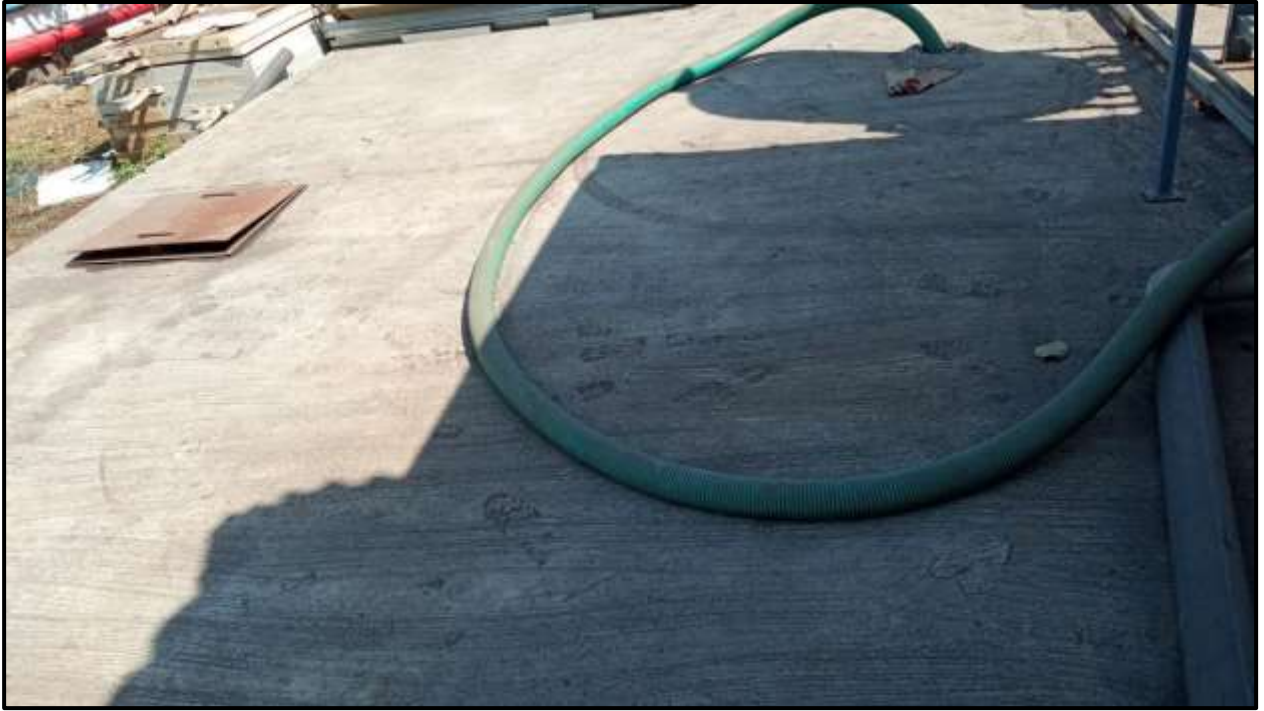
Rain water harvesting Tank
